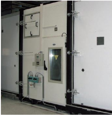
Thermal Chamber, Source: Fraunhofer, IBP
